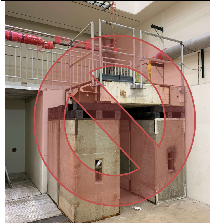
Non-rated plastic lumber utilized for a work platform support – not acceptable
